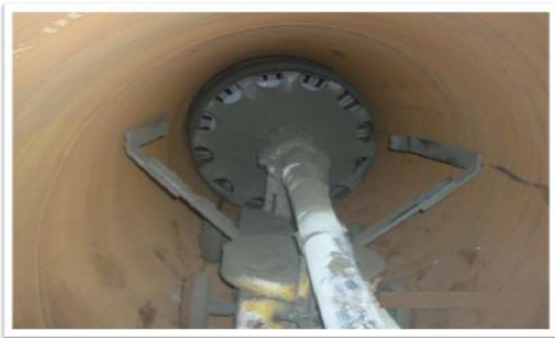
INSERTION OF TROWEL MACHINE IN TO THE PIPE FOR INTERNAL CEMENT MORTAR LINING
