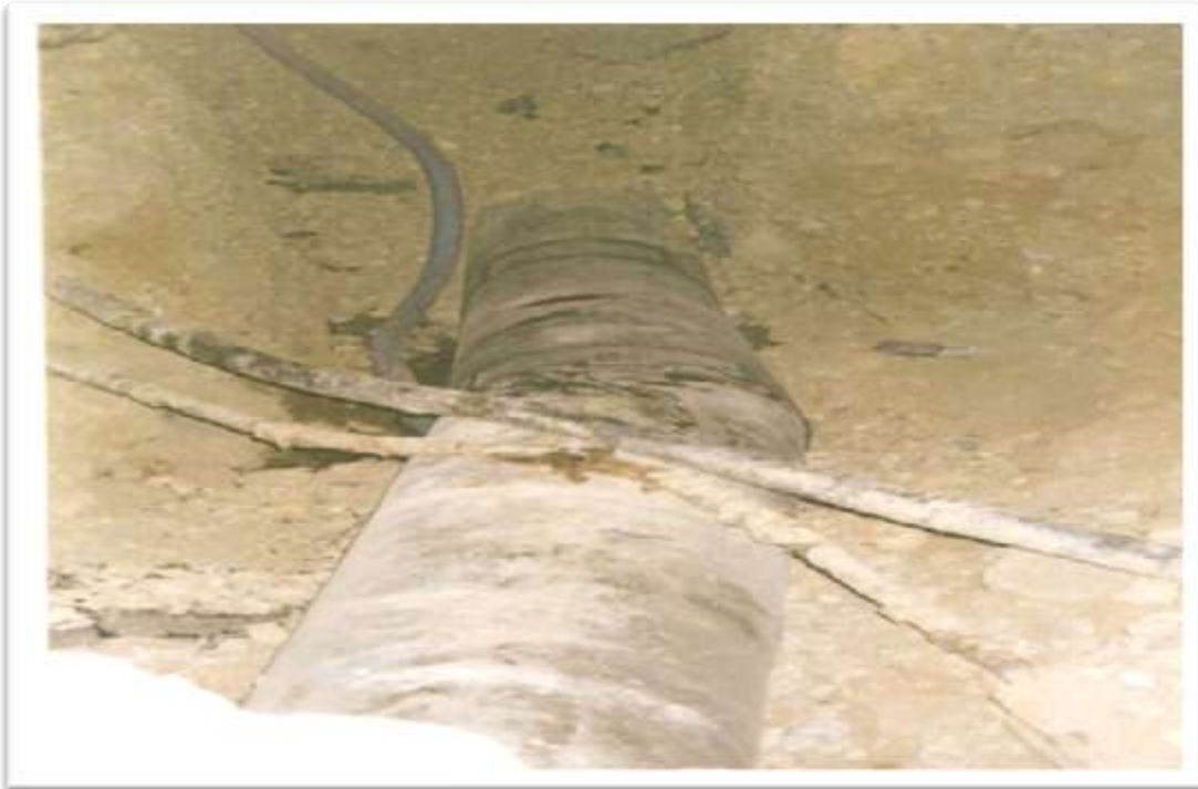
REPLACEMENT OF 24" DIA PRCC PIPELINE WITH 24" DIA MS PIPELINE UNDER GULSHAN CHOWRANGI FLYOVER
