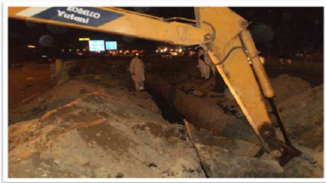
EXCAVATION IS IN PROGRESS IN NIGHT EMERGENCY WORK AT GULISHAN-E-IQBAL, SAFARI PARK
