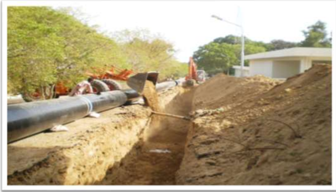
EXCAVATION AND SPREADING OF BEDDING MATERIAL WITH LOADER ARE IN PROGRESS AT SITE
