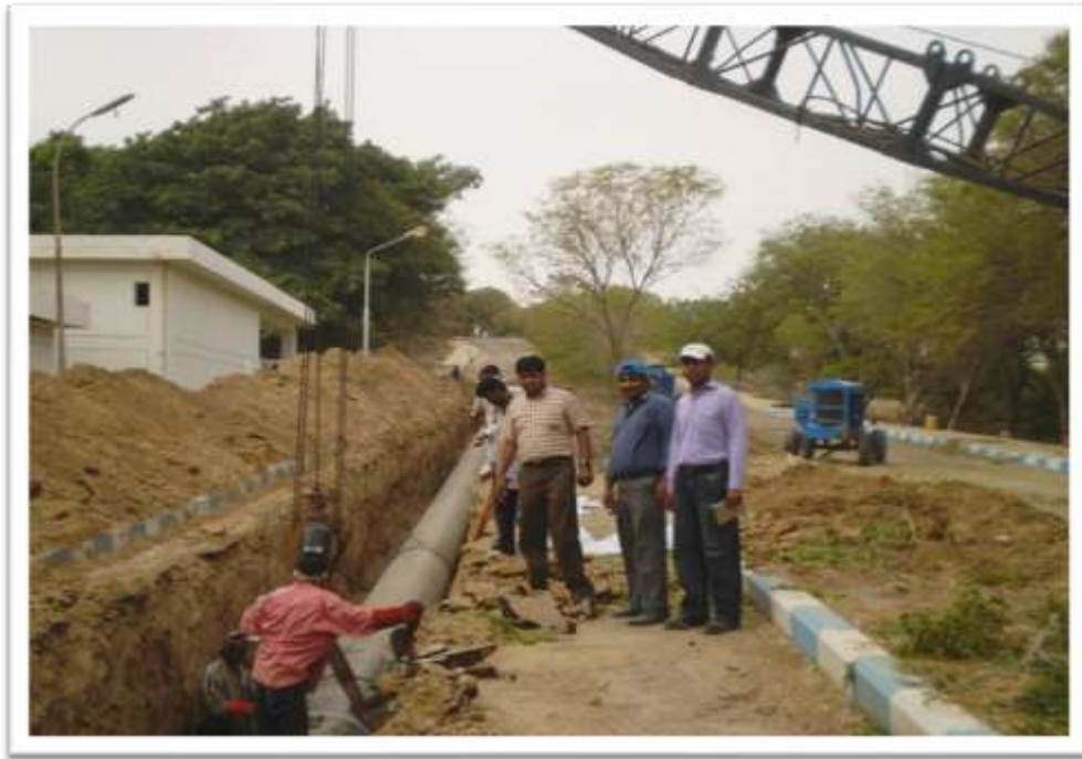
PIPE LAYING & JOINTING OF 36" DIA IS IN PROGRESS AT PIPRI FILTER PLANT
